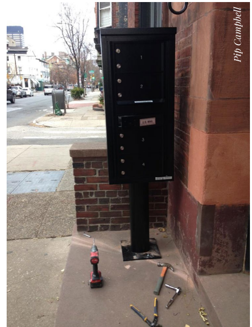
Sidewalk mailbox installed without Historical Commission compliance.
