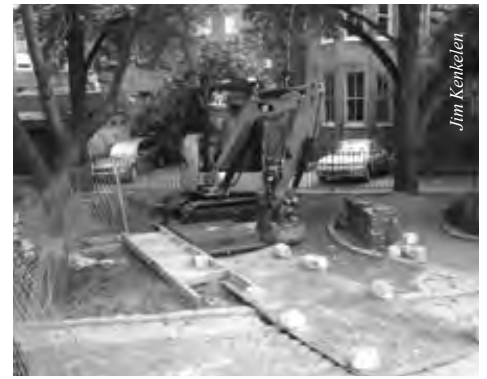
Portions of Fidler Square were dug up during the installation of the fountain's new recirculating pump system.
