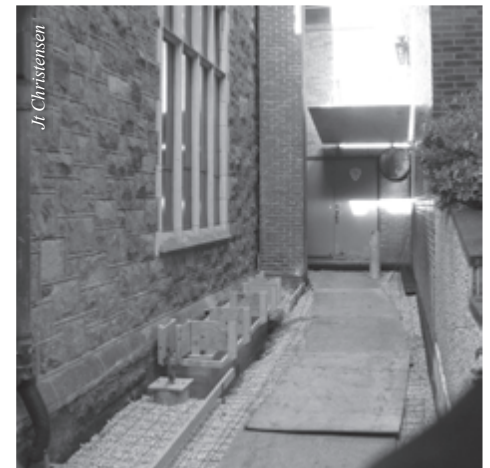
Included in the renovations being made to the 141-year old First Presbyterian Church is a new Chancellor Street entrance.
