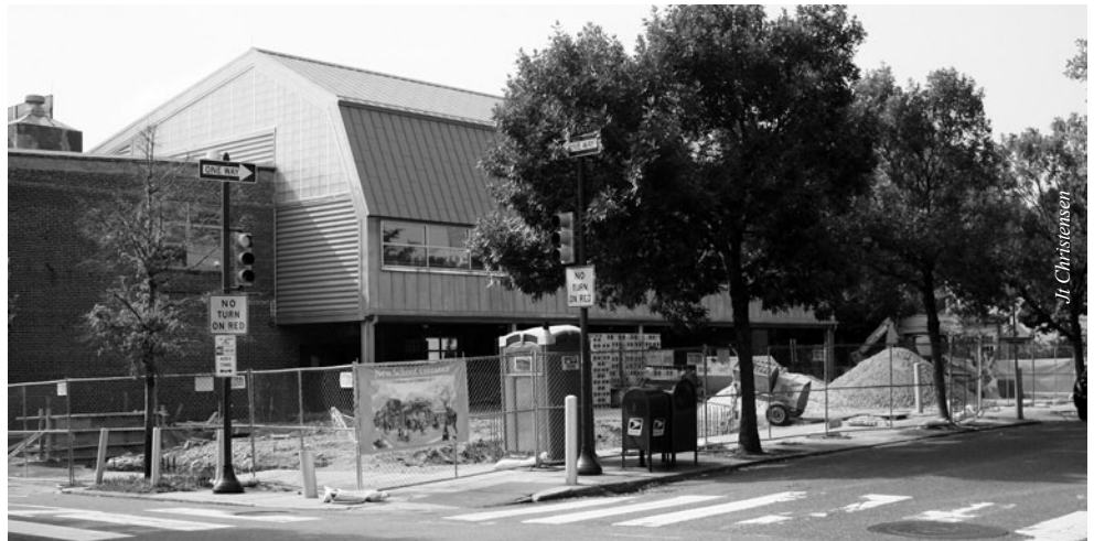
Construction began in June on the new 25th Street entryway to the Philadelphia School.
