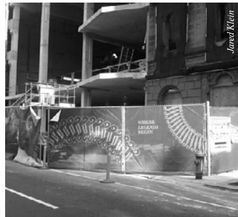
The sidewalk closure at the Curtis construction site creates problems for pedestrians, cars and SEPTA buses on the 1600 block of Locust Street.
