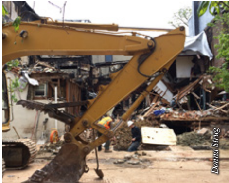
Remains of the destroyed house are visible behind backhoe being used to remove debris.
